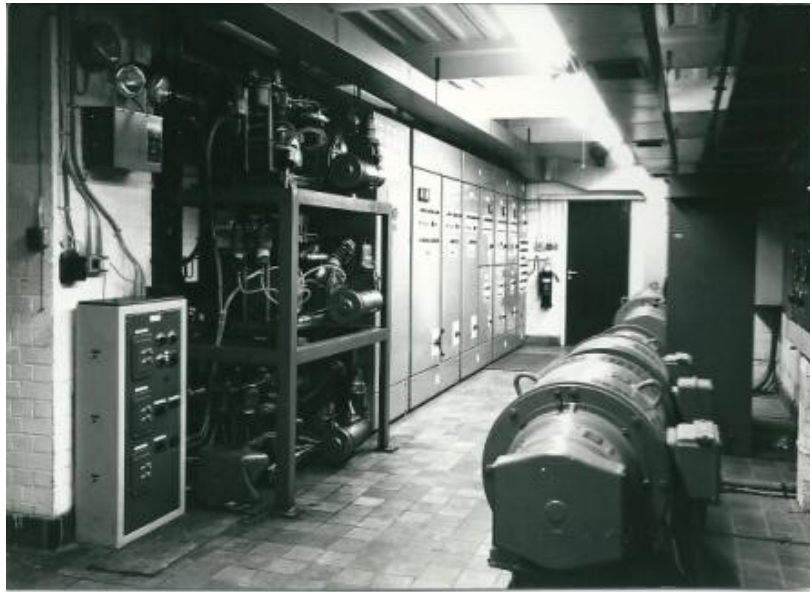
Figure 9. Motor-alternator sets and power distribution cabinets alongside the main Atlas 2 machine room at the CAD Centre.
