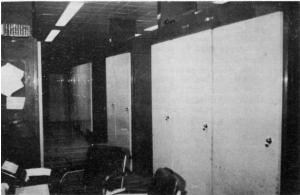
These show two more views of the cabinets containing the logic circuitry and the control circuitry in the lower room.
