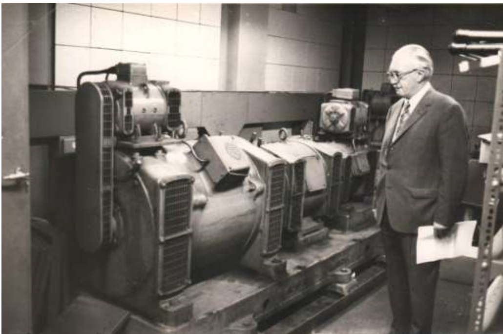
These motor alternators, of which there were three, supplied the power to the computer. One set was a stand-by. There was a separate small set supplying 80 cycle current to drive the four magnetic drums.
